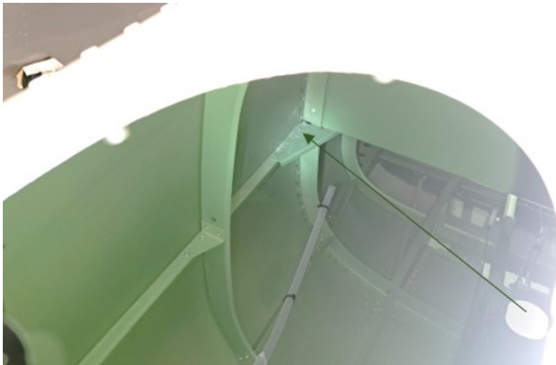
Fig. 12 Missing rivets on the left side installed through the inspection hole on fuselage bottom
